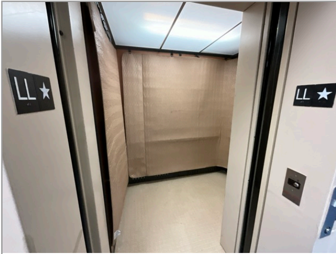
LOBBY LOOKING AT CABS (WITH DOORS OPEN)
