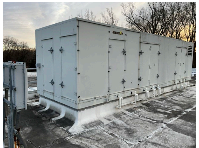
22 - ROOFTOP PACKAGED UNIT
