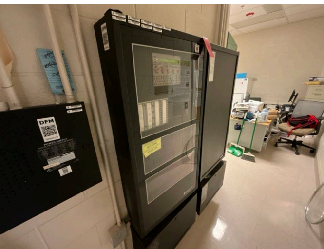
17 - FIRE ALARM PANEL
