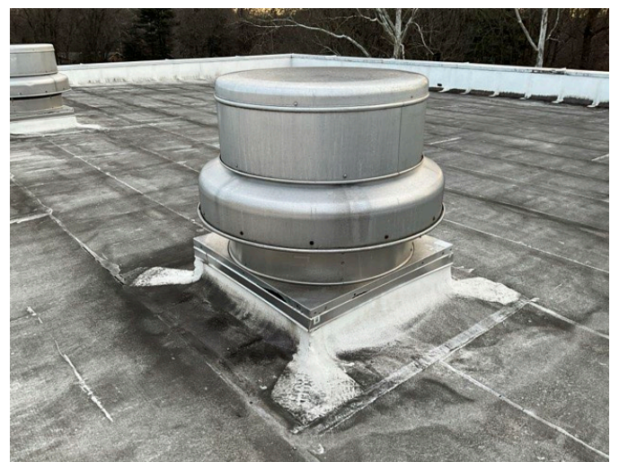
24 - TYPICAL EXHAUST FAN
